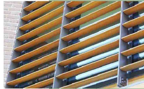
Sun shades - reduce cooling
